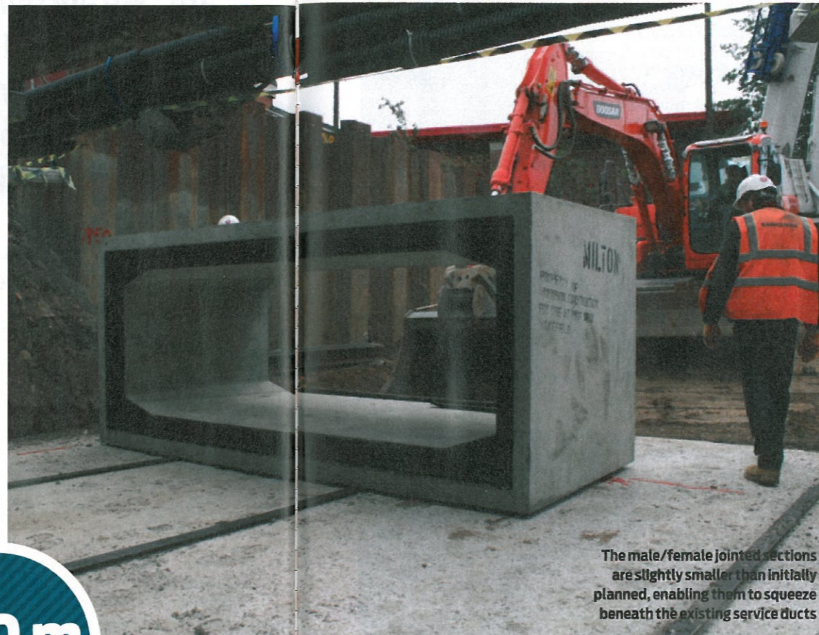
The road diversion (top) was essential to allow work on the Westgate culverts (bottom) to begin
